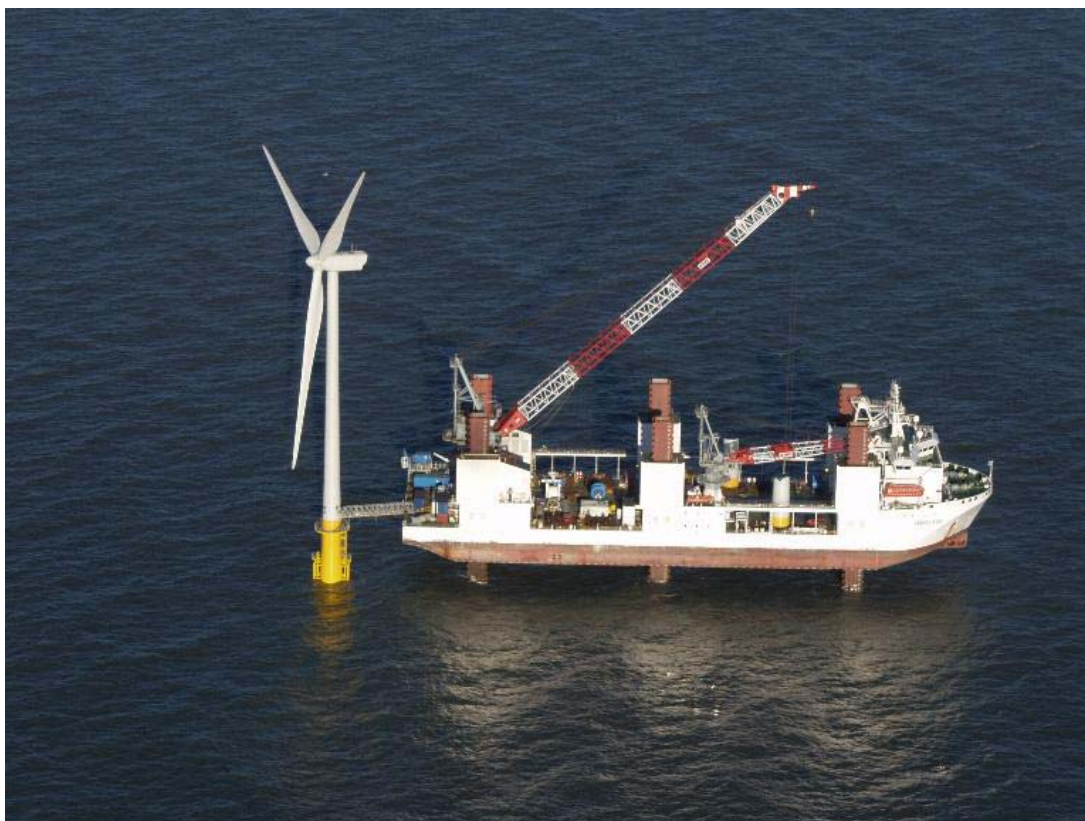
A Wind turbine under installation at Barrow Offshore Windfarm, DONG's biggest development in 2005.
