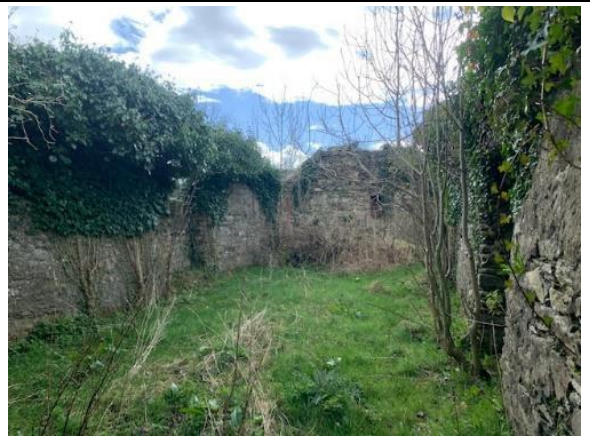
Plate AIV.8: Derelict building viewed from inside, indicated by Location 3 on the map
