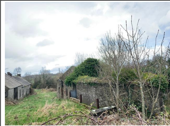
Plate AIV.7: Derelict building viewed from the south-side, indicated by Location 3 on the map
