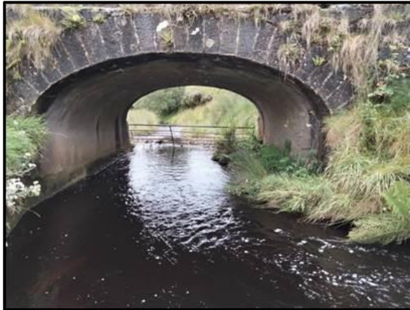
Plate A11.1.1: The road bridge over the Legnahone Burn, along the Napple Road
