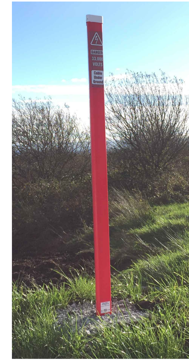
Cable Marker Post
