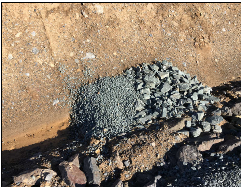
Plate 3-21: Example of a stone check dam with large aggregate on downstream side
