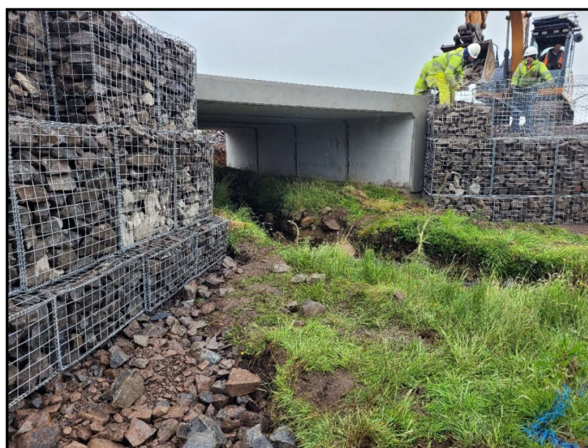
Plate 3-17: Example of a clear span pre-cast concrete box culvert over an existing watercourse
