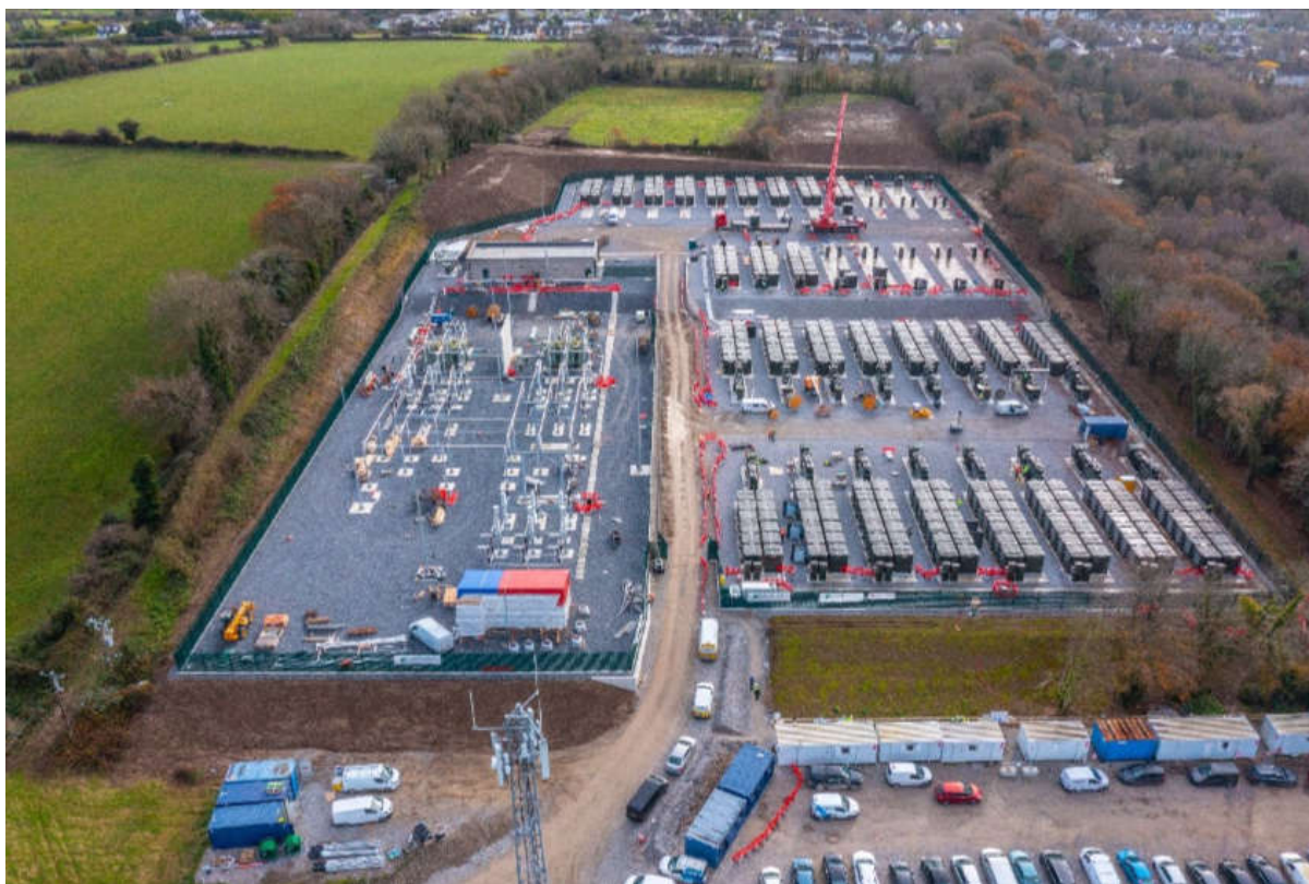
Plate 3-13: Wind farm example of a BESS Compound
