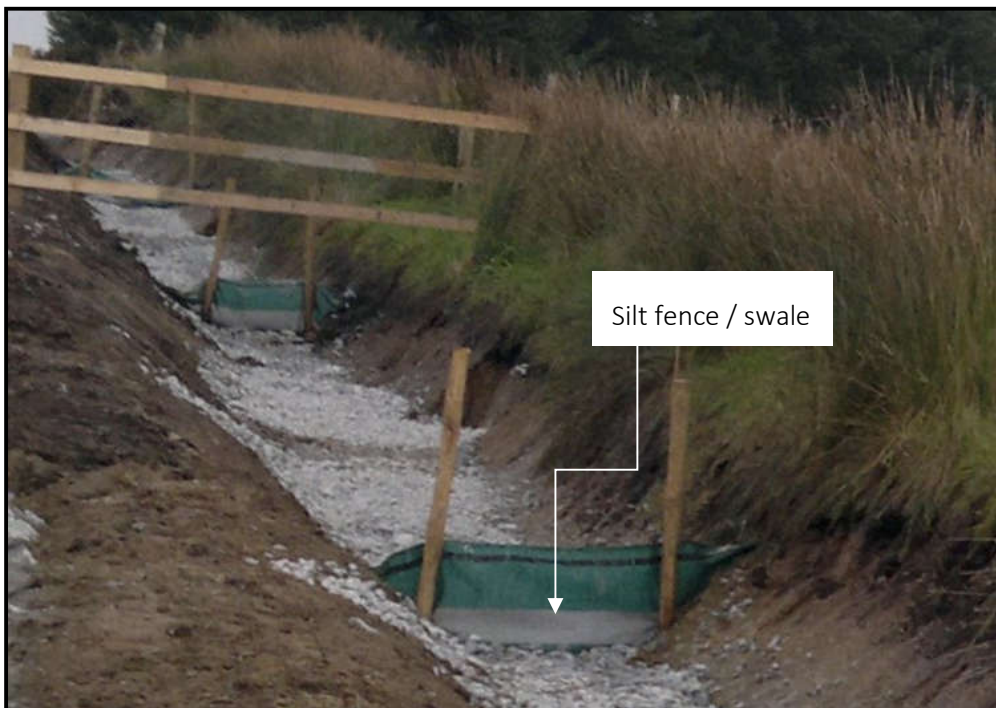
Plate 3-24: Example of a silt fence used in conjunction with check dams along trackside drainage channels
