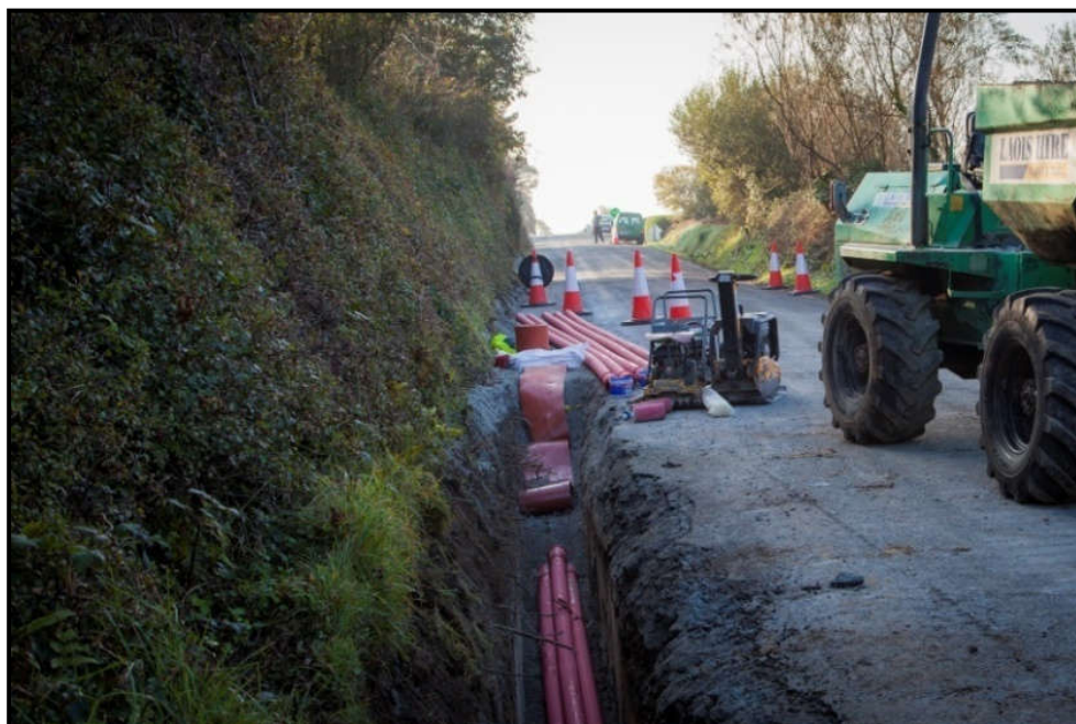
Plate 3-8: Grid Route example of the proposed ducting installation works for a cable trench
