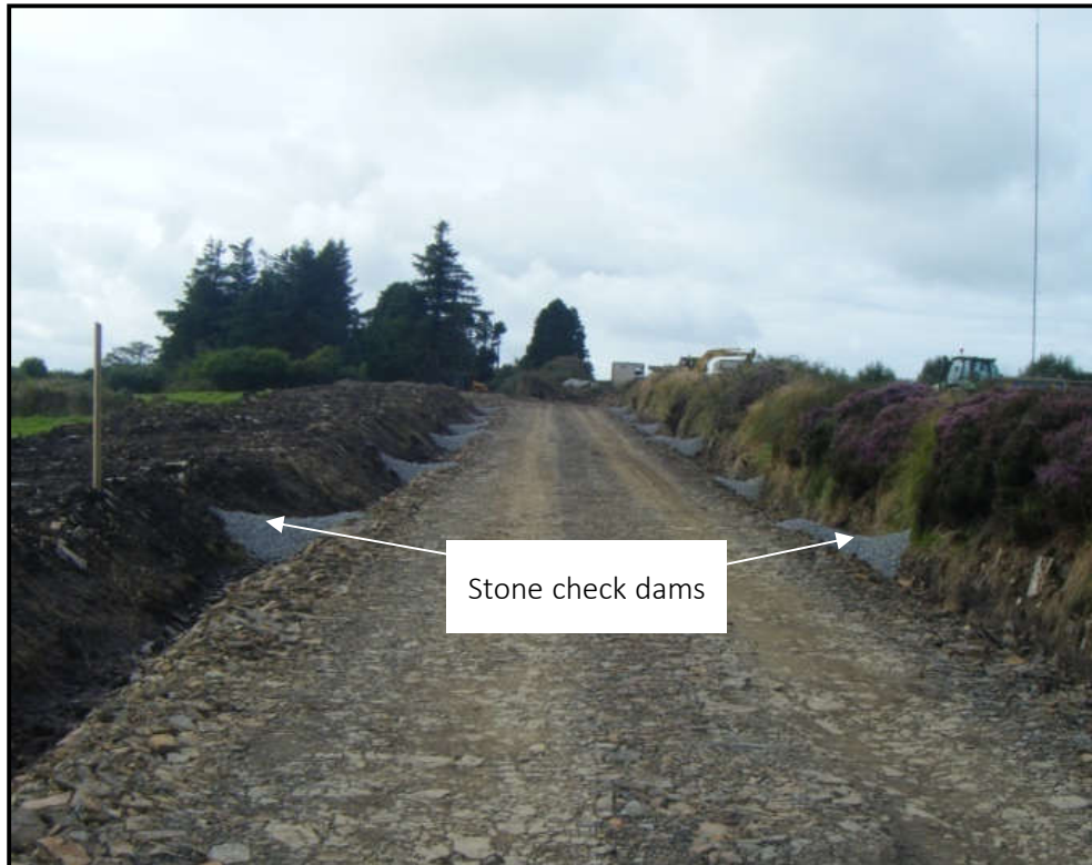
Plate 3-23: Examples of check dams along trackside drainage channels
