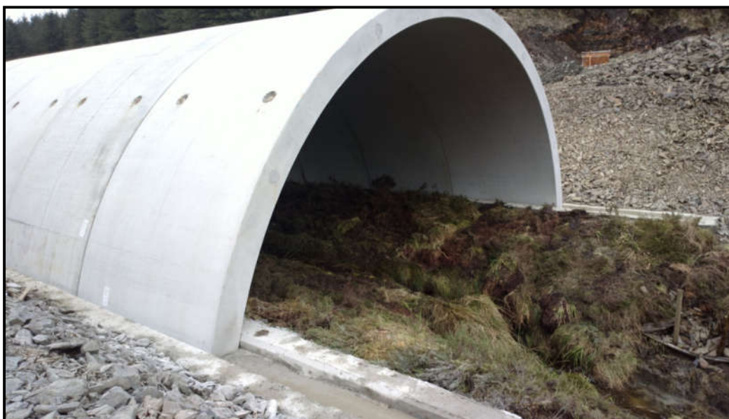
Plate 3-16: Example of a clear span pre-cast concrete arch units in place over an existing watercourse
