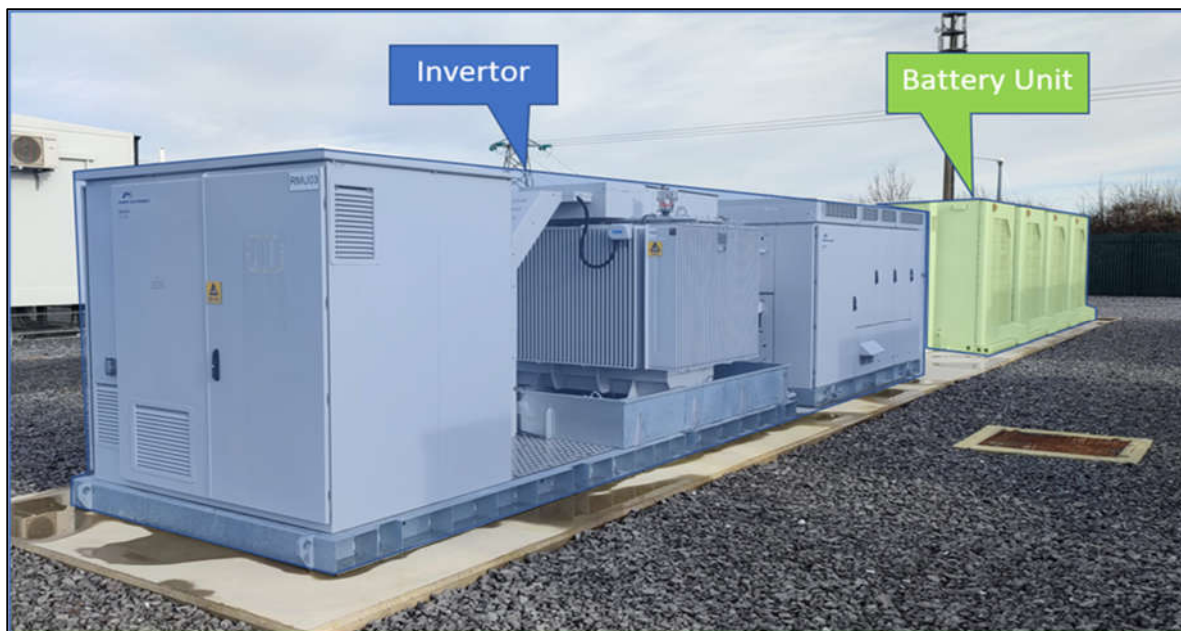
Figure 12-22. Typical Inverter and Battery Storage Units.
