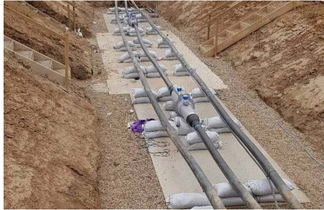
Cable joints in one of the 26 joint bays along the route
