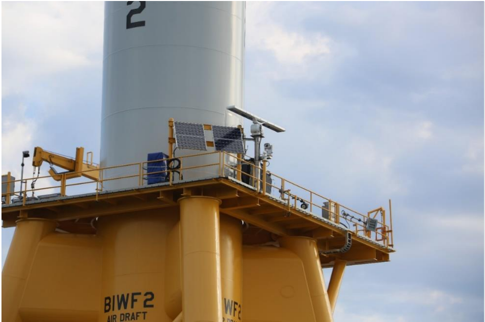
Figure 2-1 DHI’s MUSE wildlife detection system deployed on Turbine 2
